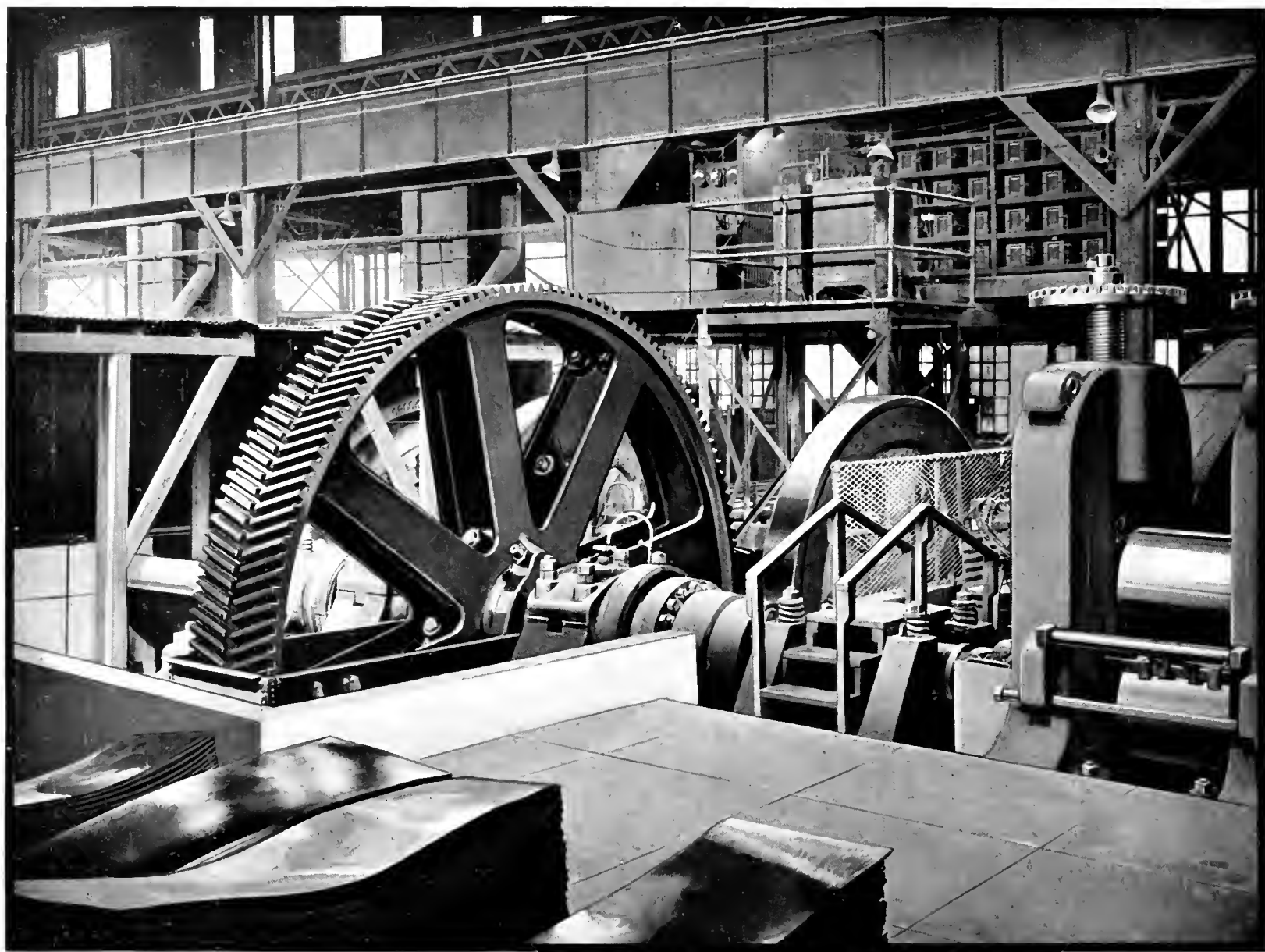
One of the Two 1200 H.P. Mesta Double Helical Cut Tooth Gear Drives Installed at the Plant of The Standard Tin Plate Company
